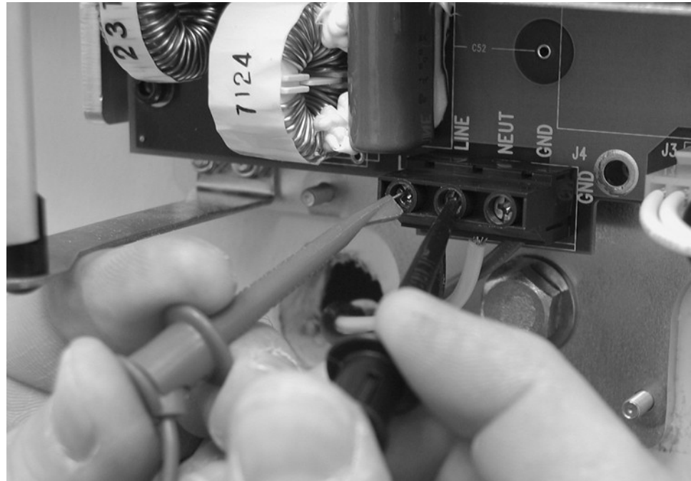
Figure 24 Verifying Input Voltage at the Line Input
